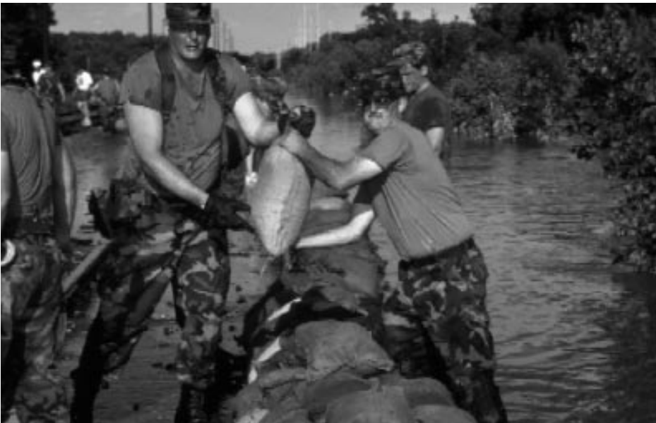
Civilian volunteers and National Guard personnel build a sandbag levee at Valley Junction, Iowa, trying to stop flooding of the Raccoon River in July 1993.
